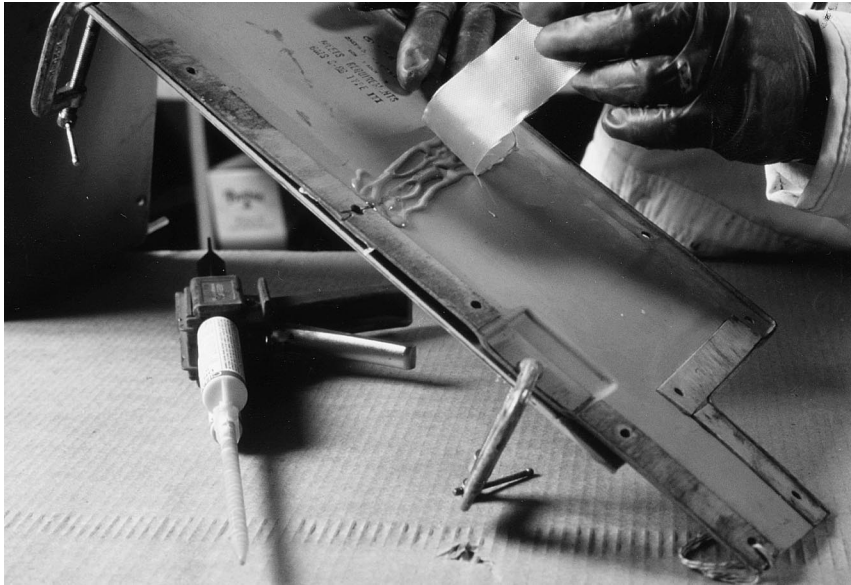
Fig. 4. Additional adhesive is dispensed around the panel's surface and then a fibreglass doubler is placed over the area surrounding the crack.
