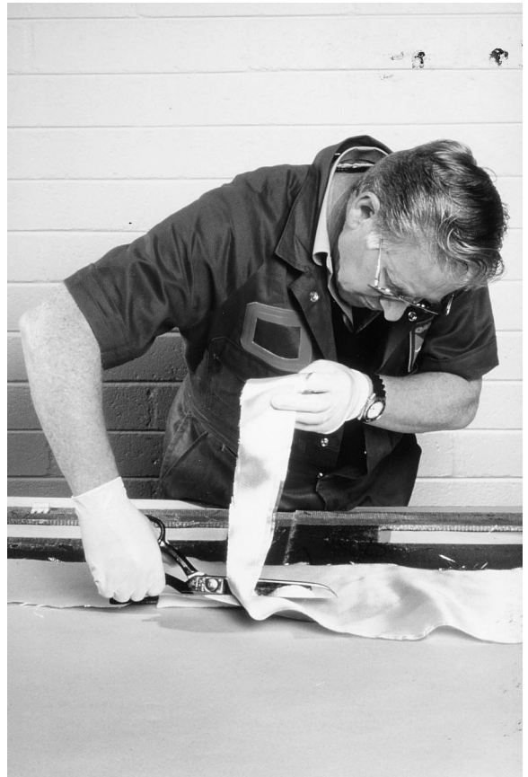
Fig. 14. After removing damage and solvent wiping the panel, several fibreglass plies are cut to fit the repair area.
